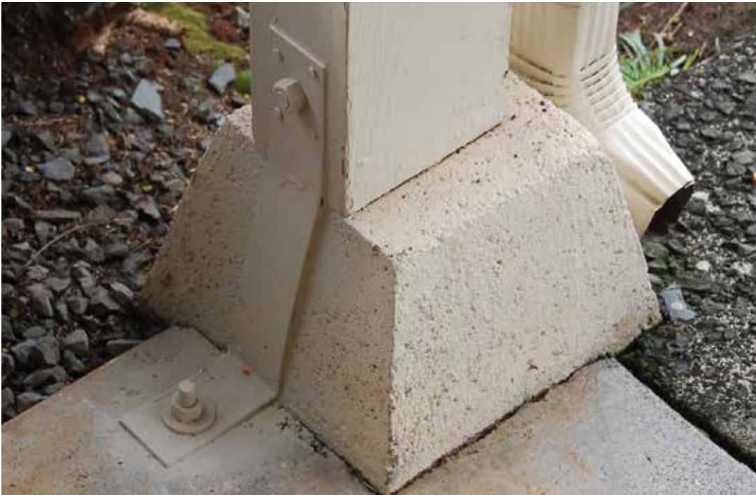
Figure 2.13. In some retrofit examples, it is possible to tie a portion of the house to the foundation. Here, a metal strap connects the vertical post to the foundation, which attempts to finish the continuous load path connection from the roof to the foundation. The strap has been primed and painted. Source: Hurricane Protection Services.
