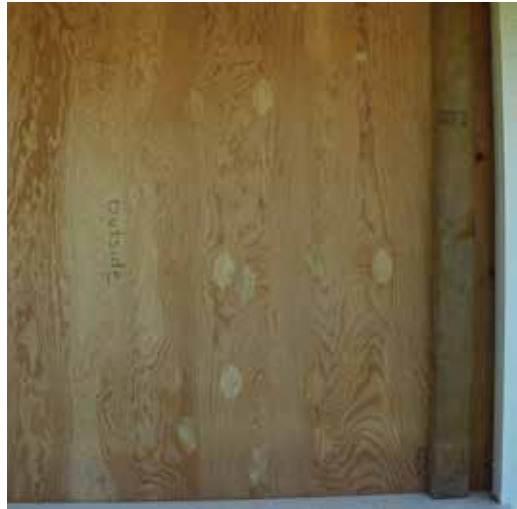
Figure 2.26. The joint between the plywood is short, for example 4 feet to 5 feet in length, a 2x4 can be used with the wide end on the outside against the plywood. Both ends of the 2x4 are then attached with screws through the plywood and into the window frame. This will require two 4 inch or 4.5 inch lag screws which may require pre-drilling. Source: Figures 2.26- 2.29, University of Hawaii Sea Grant.
