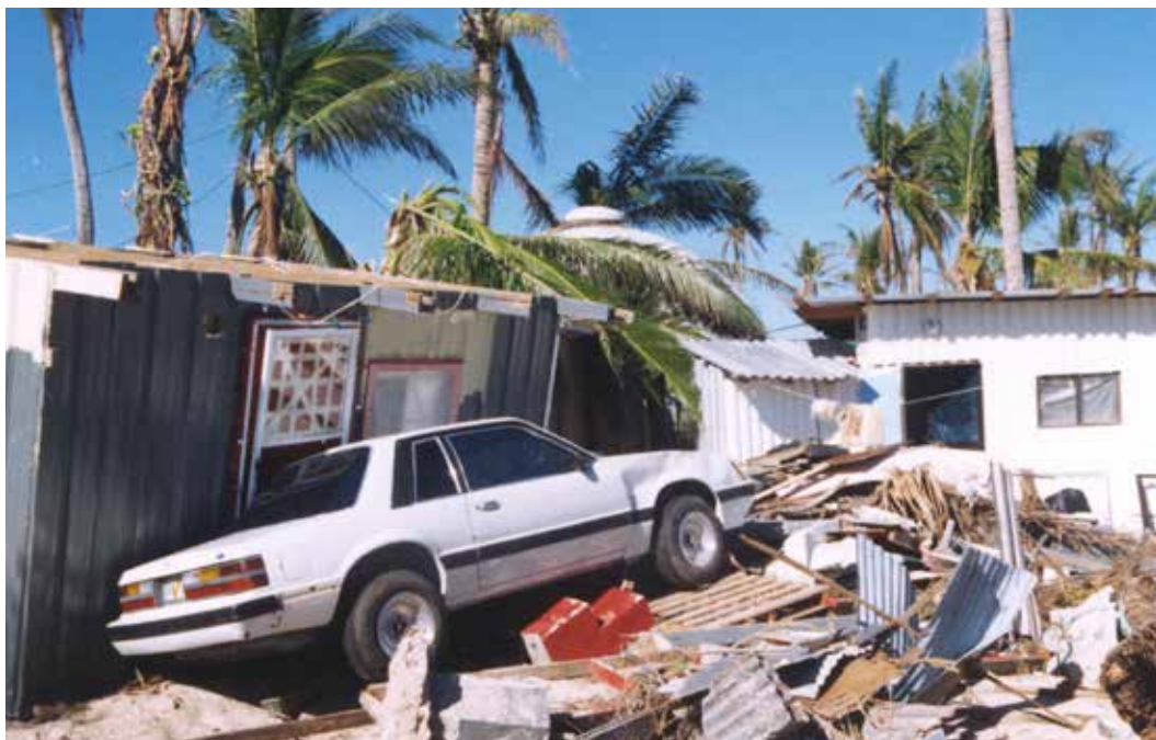
Figure 3.3. A home in Dededo was damaged after Typhoon Paka in 1997. Source: FEMA.
