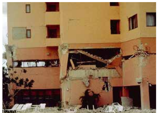
Figure 1.1. Damage to the Royal Palm Resort Guam, a new 12-story hotel and condominium complex, after an 8.1 earthquake on Aug. 8, 1993. The building collapsed just 18 days after opening. Source: FEMA.
