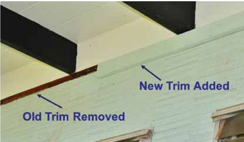
Figure 2.19. The old trim has been pulled off. The new trim is 1 inch by 4 inch exterior wood, treated for termites, painted with primer and two coats of paint that match the wall. Color matching can be done by taking a small sample to your local hardware store.
