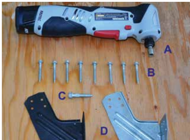
Figure 2.16. For the installation above, a right angle impact driver (A) is used to install the manufacturer's specified connections. Eight \frac{1}{2} inch length screws (B) are used for the top tab and bottom tab. One \frac{1}{4} inch 1\frac{1}{2} inch long screw (C) provides connection from the trim board to the wall. The HPT clip (D) is also shown.
