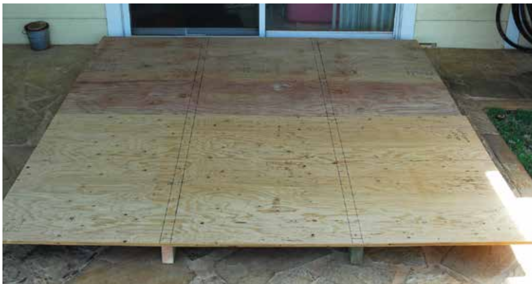
Figure 2.28. During the assembly of the larger shutters like those used on a sliding glass door, the two panels to be joined sit atop 2x4s. The outline of the 2x4s and all screw locations are marked on the panel. Panels should be cut, labeled and marked as to all fastening locations before a typhoon is on the way. The panels can be quickly attached with wood screws drilled from the plywood panel into the 2x4. The panel is then lifted up and attached to the structural frame of the window.
